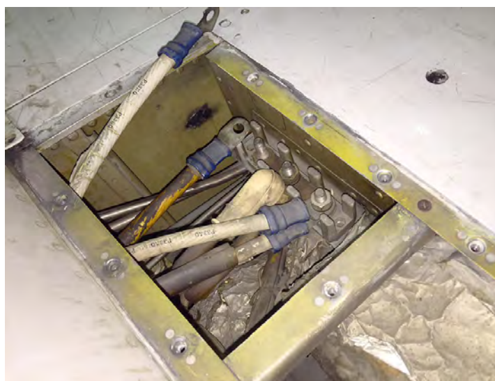
Beech. External Power cables disconnected at Terminal Strip.
