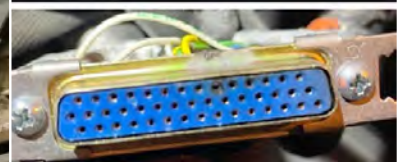
Left: IFE wiring cannon plug with burnt connections.
