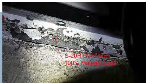
Right: Bombardier. Close-up of corrosion.
