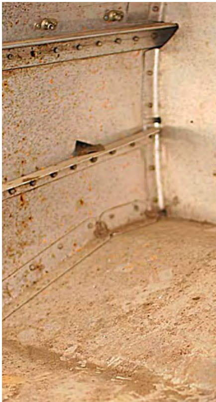
Above: Direct chemical attack in a battery compartment.
