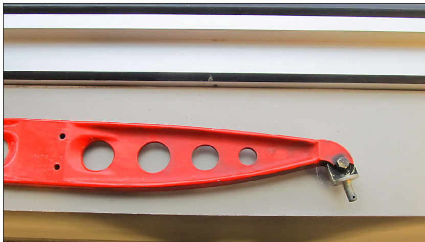
Douglas-Hinge with missing piece.
