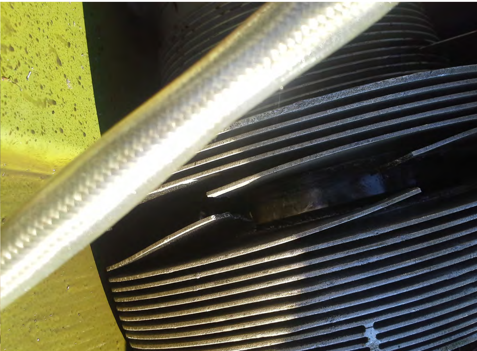
Opposite: Garrett. Rotor assembly with rivets that had fallen out due to incomplete setting. Above: Teledyne. Cylinder with obvious head separation.
