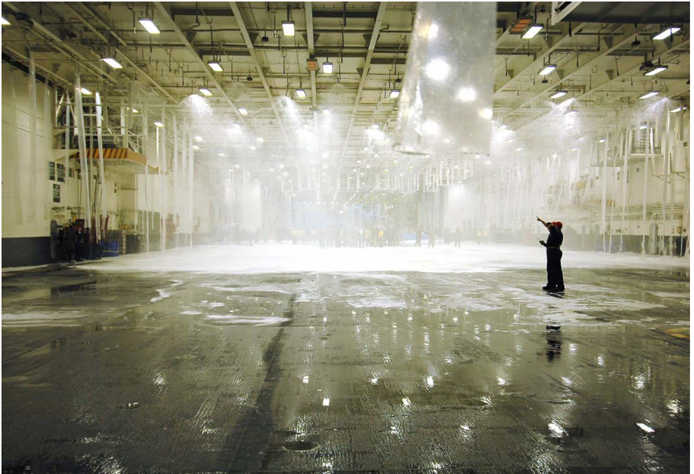
Above: Hangar-Staff observe aqueous film forming foam (AFFF) fire suppression system in action.
