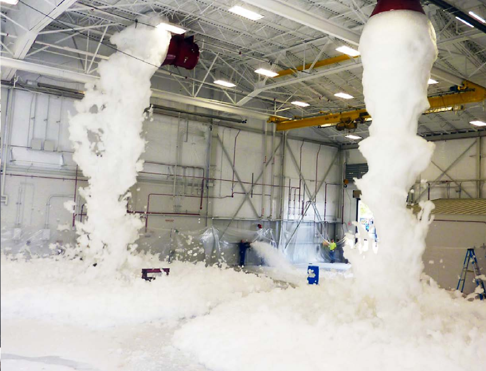
Opposite: Aircraft support apparatus can be in different areas in a hangar at any time, and contain possible fire ignition sources. Above: The fire suppression system discharges foam at a rapid rate.
