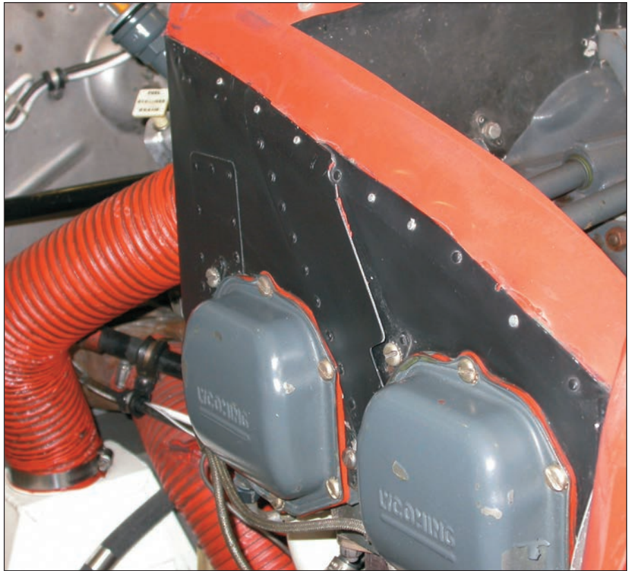
Properly maintained engine baffles and seals are essential to engine cooling and operation.
