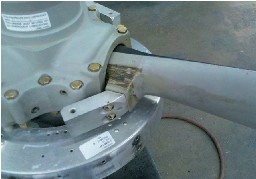
A common blade grease leak caused by over-greasing.
